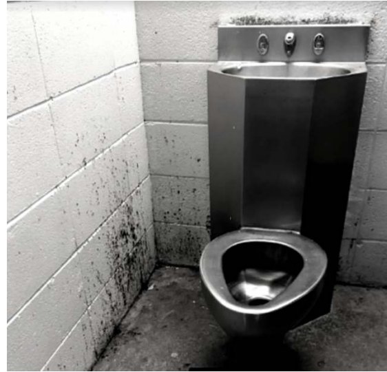
Figure 6: Photo of mold in Camp J shortly after camp closure
